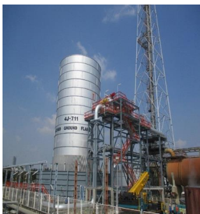
Bangchak Enclosed Ground Flare (EPC)
