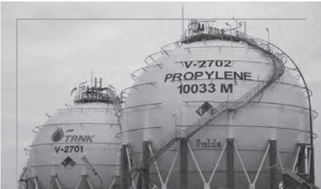
Project : PTT Tank Terminal Propylene Spherical Tank Propylene Storage 4,000 tons.
