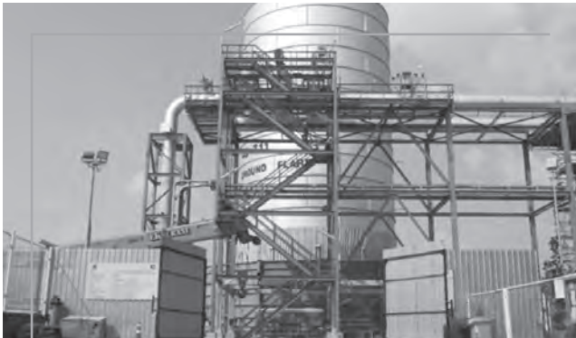
Project : BCP Enclosed Ground Flare (EGF).
