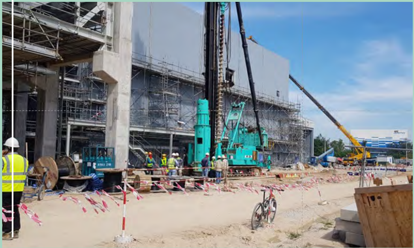
PTTLNG Receiving Terminal Nongfab Project, 28" Interconnecting Pipe Line (Piping)
