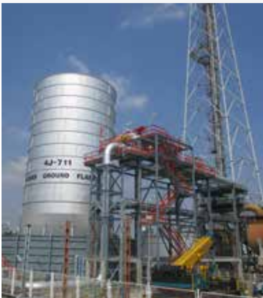
▲ BANGCHAK Enclosed Ground Flare (EPC)
