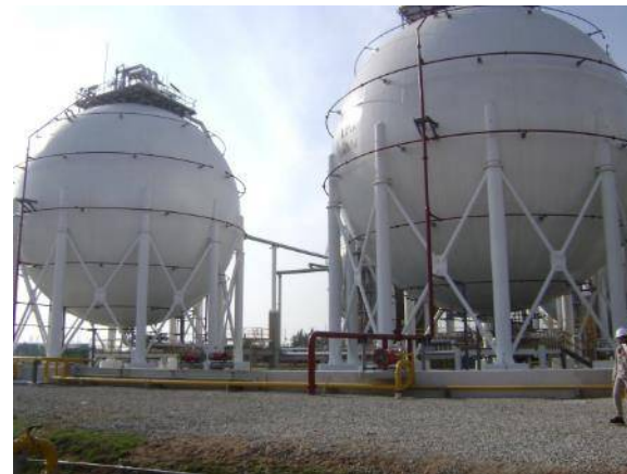
PTT LPG Tank/ Kaoboya
