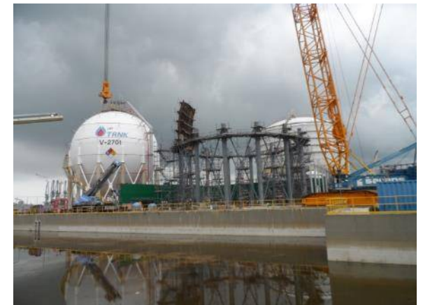
PTT Tank Terminal PP Tank
