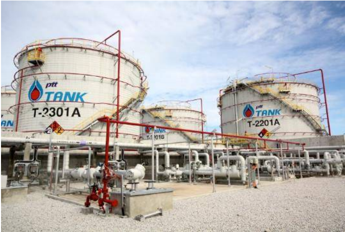
PTT Tank Terminal
